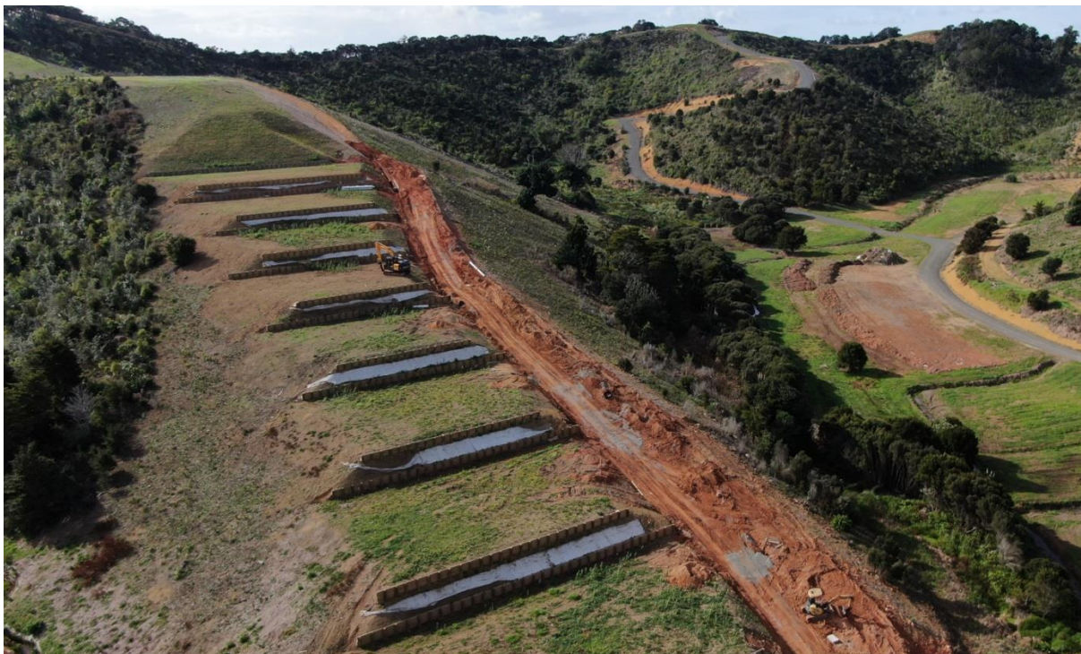
Figure 2 - Lot 1 and Lot 2 during the construction phase. Note the location of the retaining walls and batters on the left and right-hand sides (west and east). Source CES Ltd.
